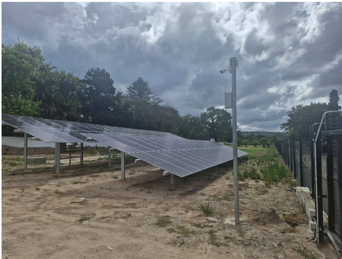
Figure 5: The same solar facility on Vredenburg farm as a visual example.
