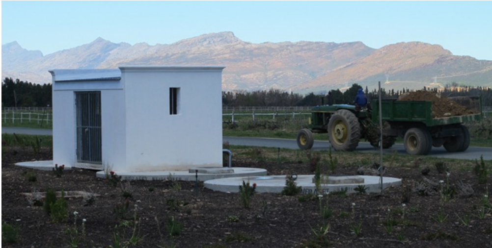
Control room built above bioreactor
