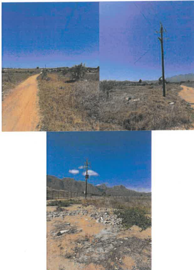
Figure 4: Existing Eskom Electrical Infrastructure
