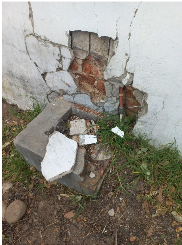
Figure 35 plaster delamination due to the previous use of unsuitable plaster.
