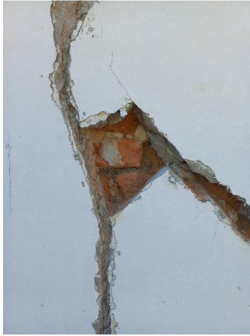
Figure 37 External wall crack and scraped cement plaster
