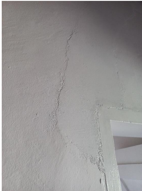
Figure 39 internal plaster crack
