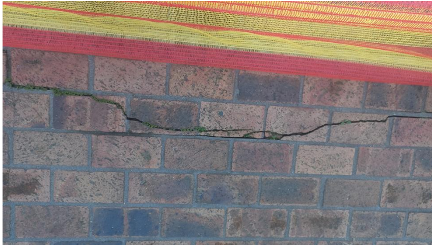
Figure 46, 47 & 48 - cracks of the stoep unreinforced slab showing on the brick paving surface
