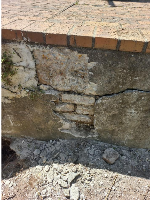
Figure 46 – stoep wall collapse
