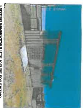
EXISTING GENERATOR AND FIRE PUMP
