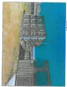
EXISTING GENERATOR IN STRUCTURE FOR EXTING FIRE PUMP - EXISTING STORAGE TANK FOR FIRE WATER
