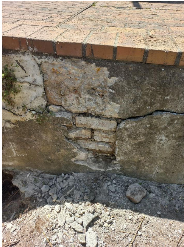
Figure 46 – stoep wall collapse
