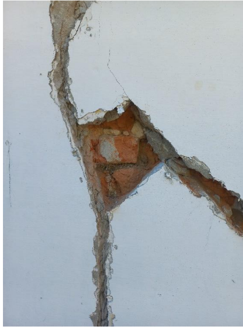
Figure 37 External wall crack and scraped cement plaster
