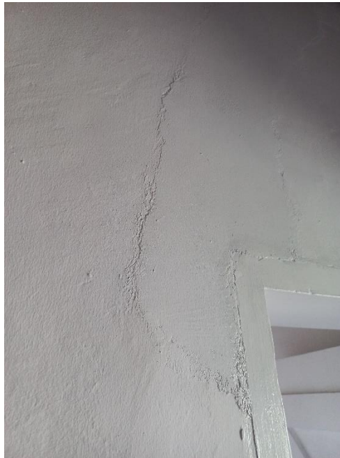
Figure 39 internal plaster crack
