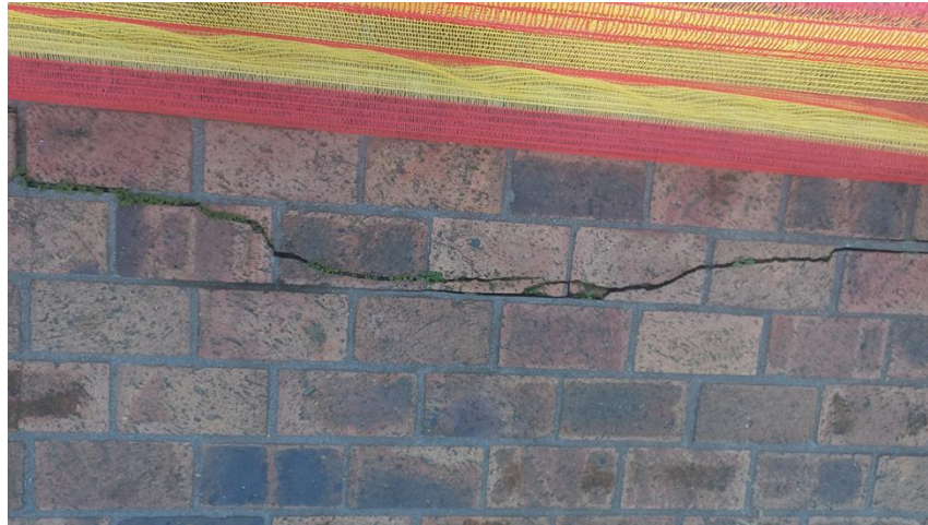
Figure and 46, 47 & 48 - cracks of the stoep unreinforced slab showing on the brick paving surface
