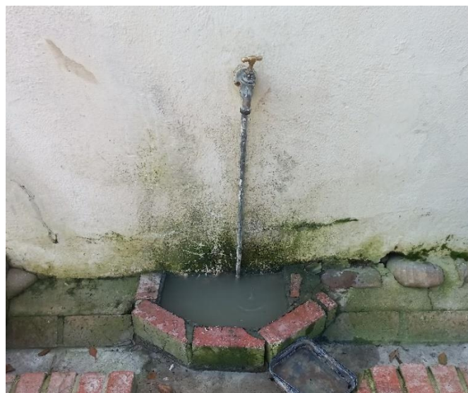
Figure 8 External tap has been relocated, since it was part of the problem,
