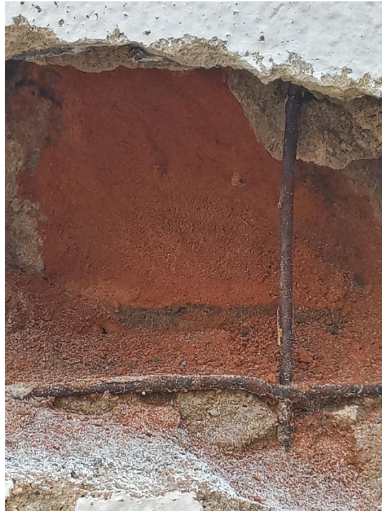
Figure 34 the inappropriate method found: wire mesh and cement plaster
