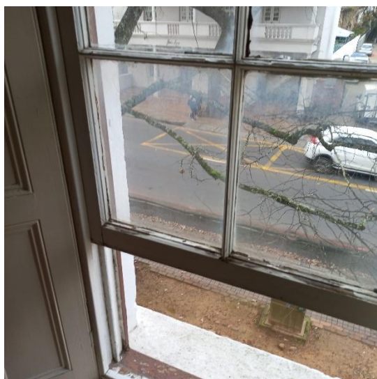
Figure 30. The state of disrepair found comprised peeling of paint, broken beads,
