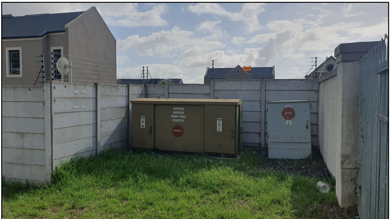
Figure 3: The electrical substation on Erf 1990, Klapmuts
