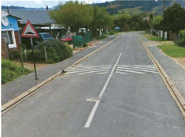
Speed hump along Skool Street
