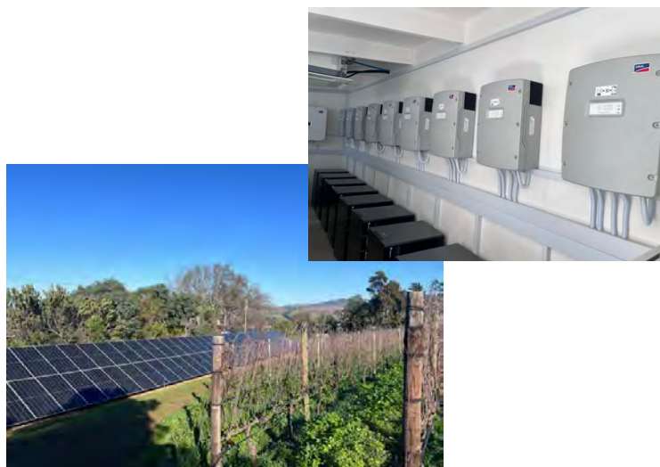
• Solar Infrastructure with inverters + batteries
