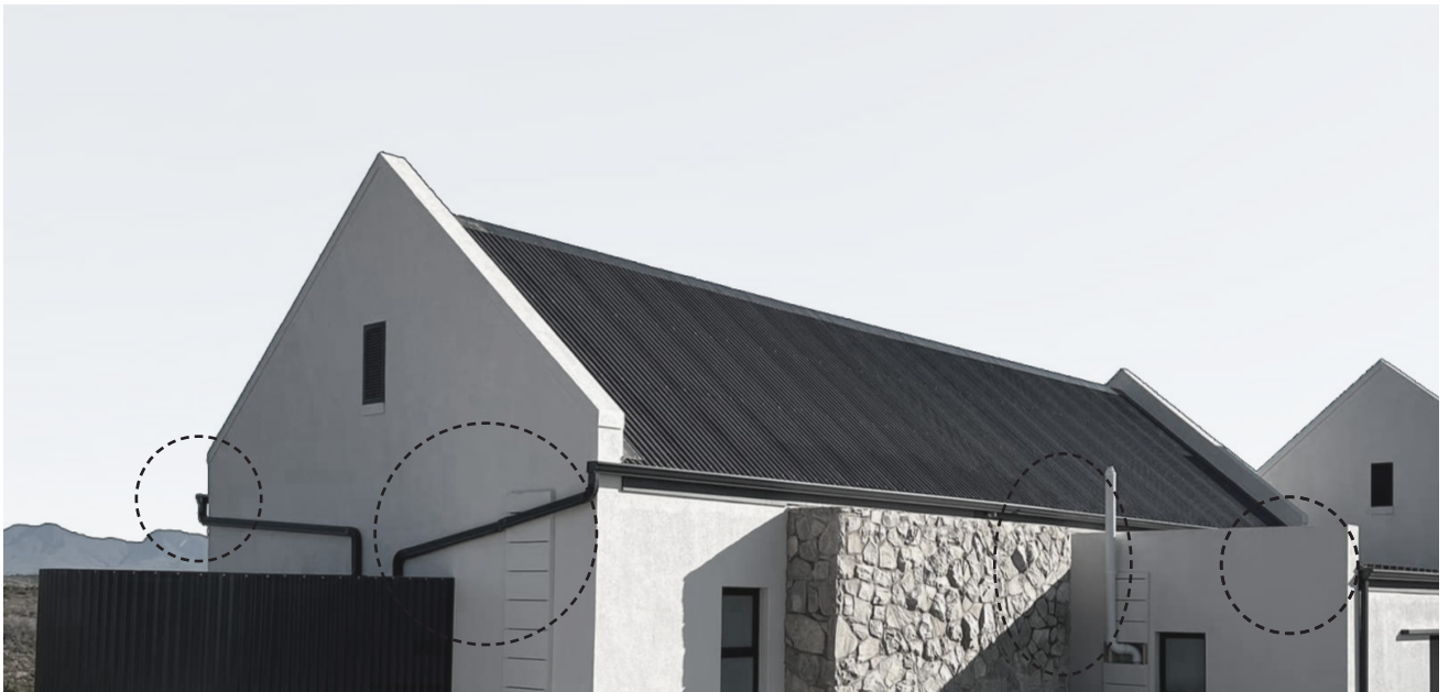
Figure 10: Good fundamentals but poor execution
