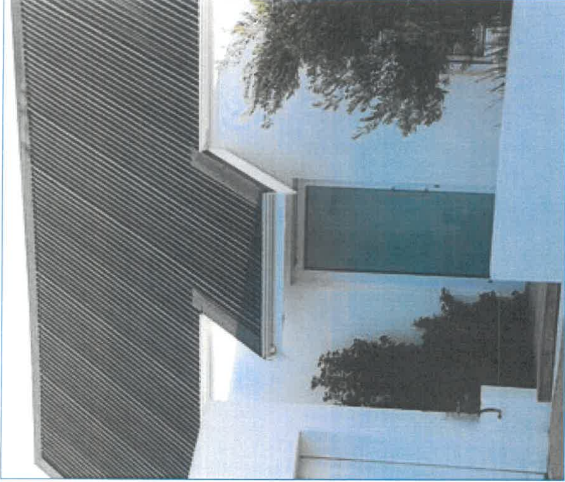
Figure 5: Entrance roof structure not permitted
