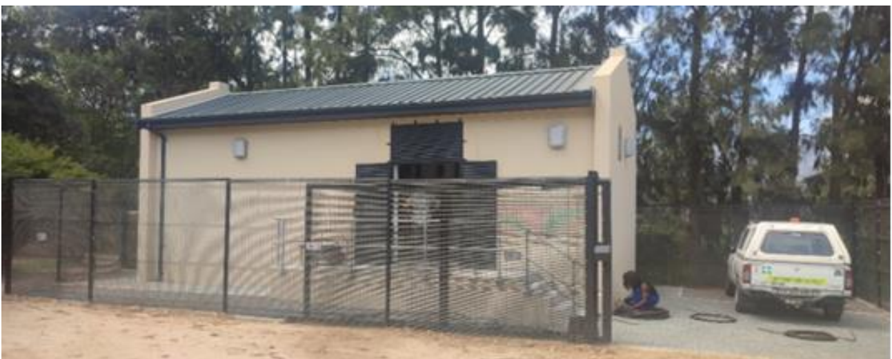
La Terra 11kv Switching Station
