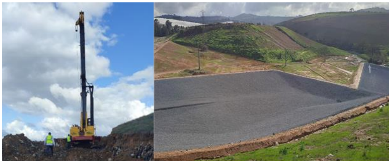
Landfill Gas Extraction and Flaring Infrastructure
