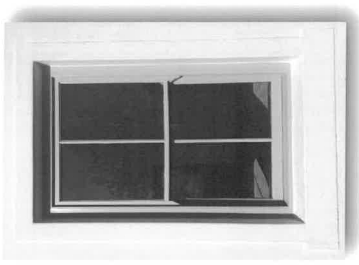
Figure 35: Plastered windowsill and plastered bands
