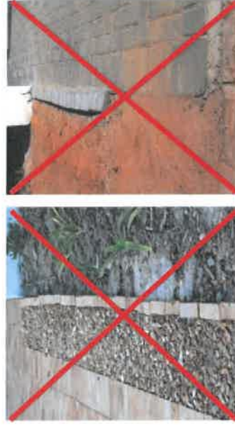
Figures 52 & 53: Incomplete and unevenly laid edging
