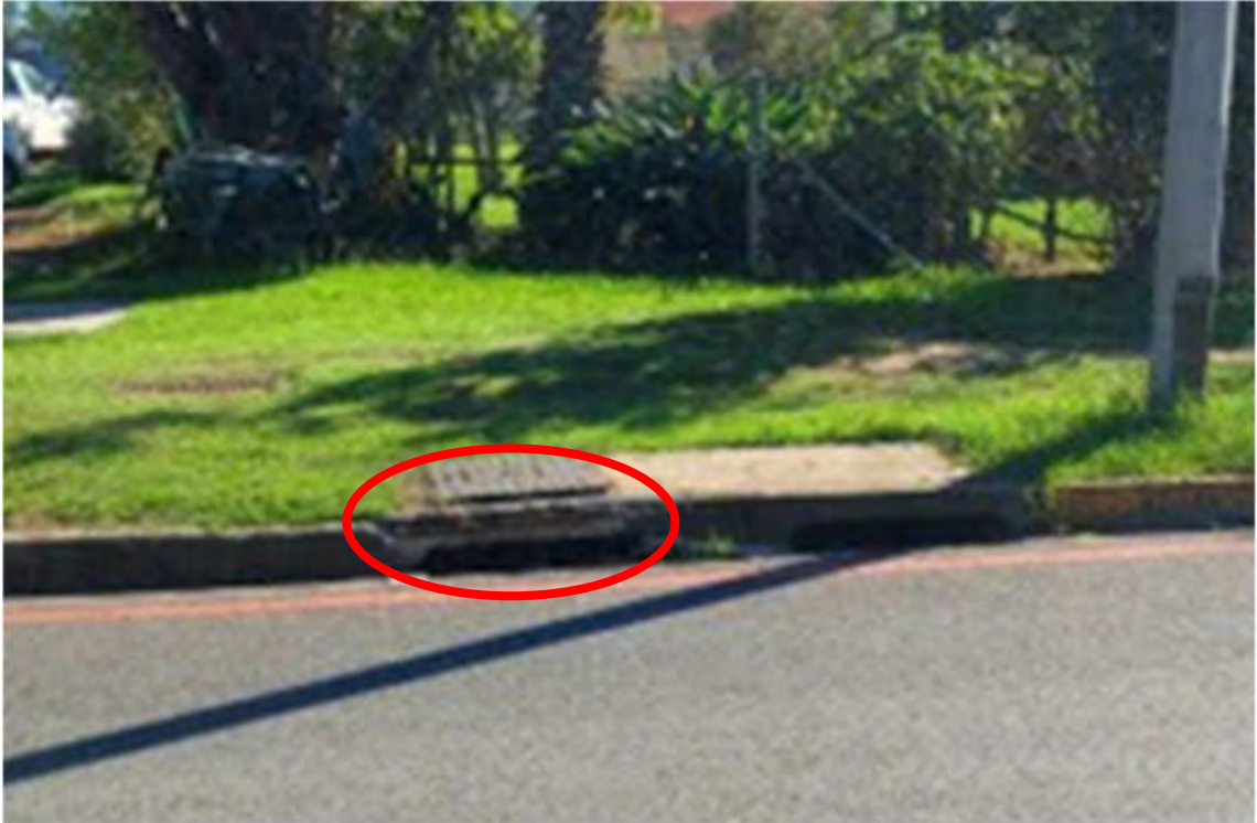
Figure 5-1: Damaged drainage channels and kerb inlets
