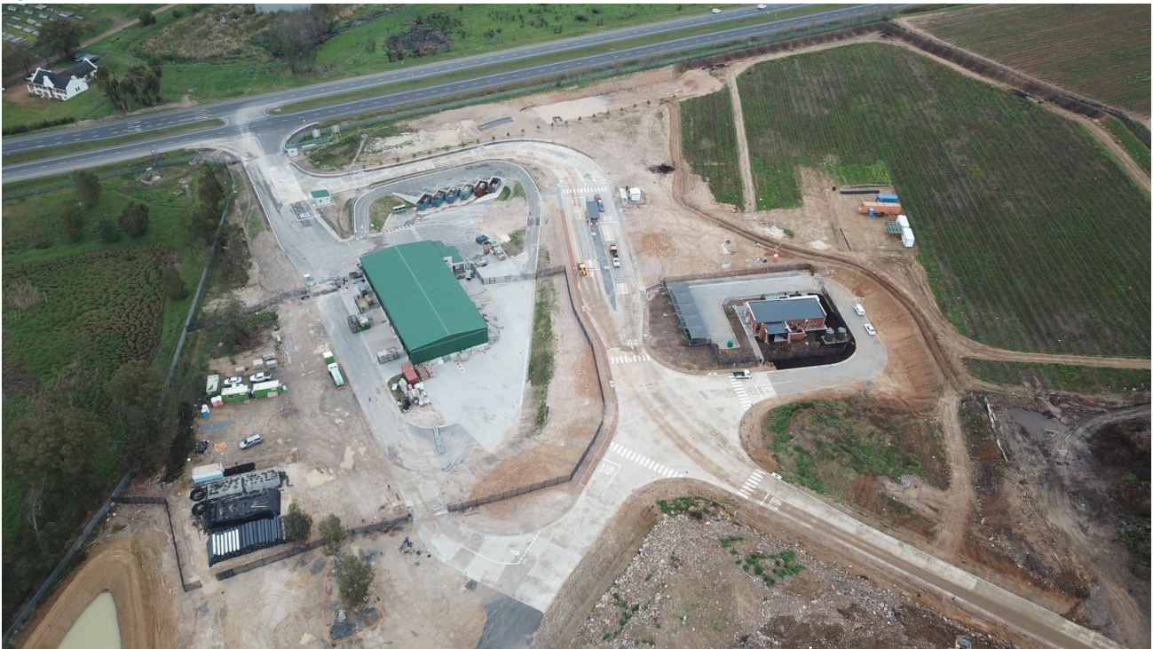
Figure 14: Material Recovery Facility (MRF)
