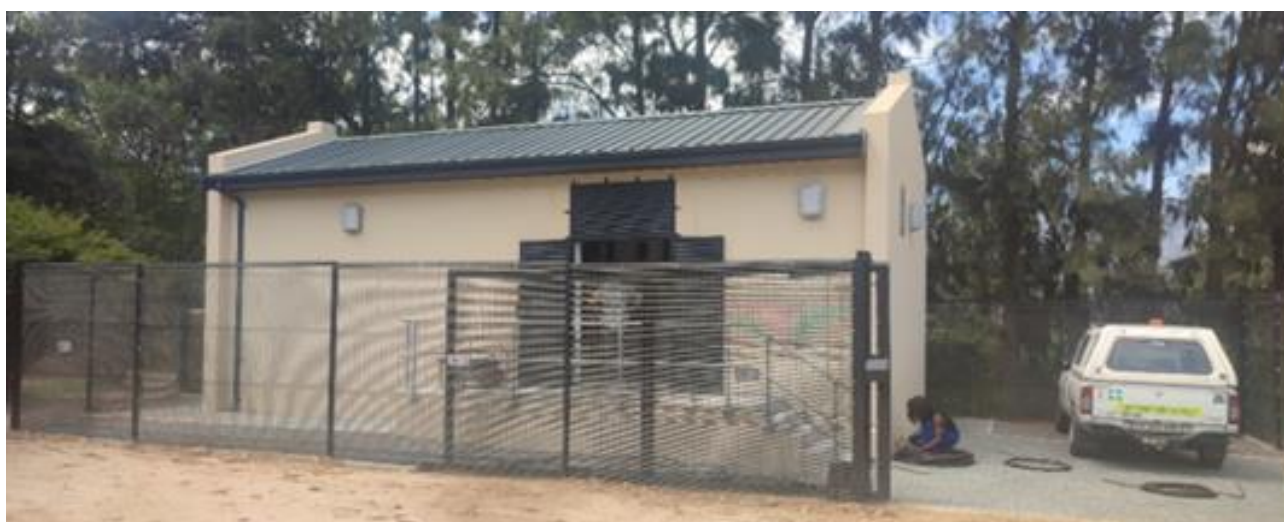
La Terra 11kv Switching Station
