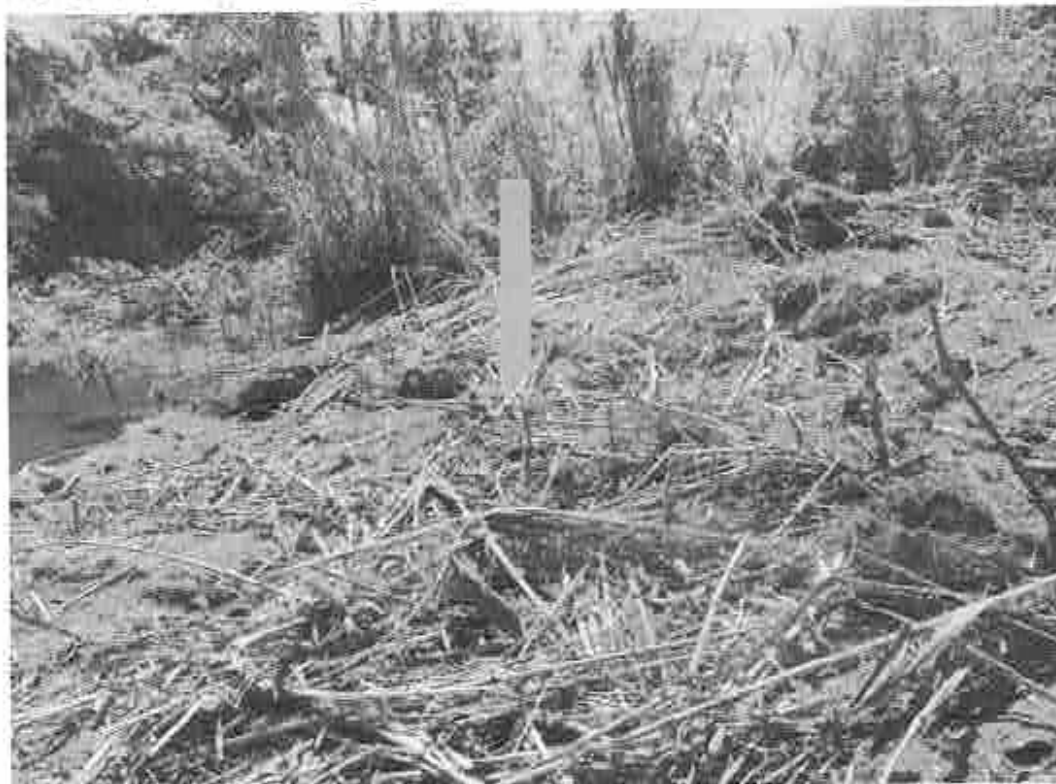
Photo 6: Evidence of earthmoving and working within the river (indicated by yellow arrow).
