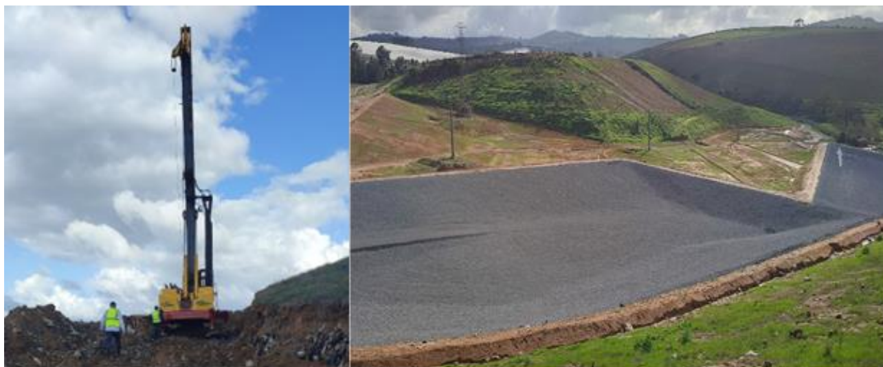
Landfill Gas Extraction and Flaring Infrastructure
