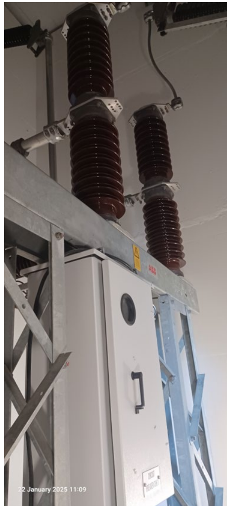
Figure 8-1: HV Circuit Breaker Located Indoors
