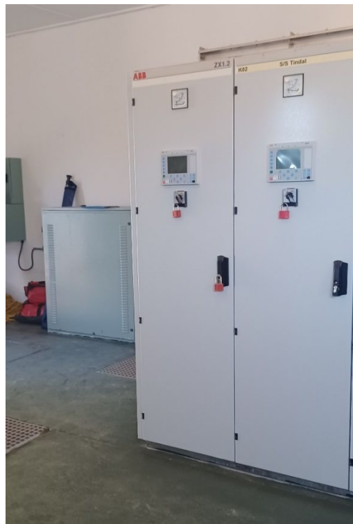
Figure 5-3: ABB ZX 1.2 panel
