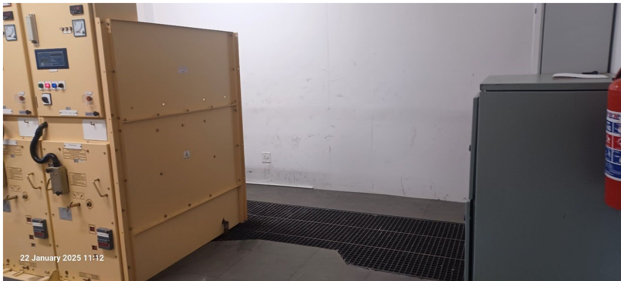
Figure 8-2: Space for Additional Panel on the switchboard Right Hand Side
