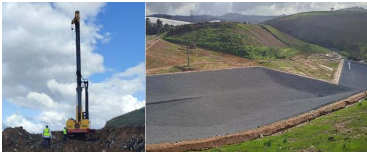
Landfill Gas Extraction and Flaring Infrastructure
