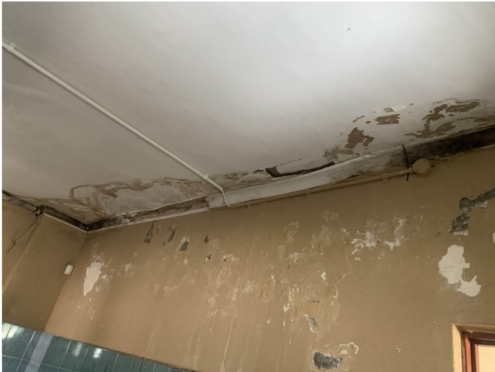
Figure 7: Ceiling and walls that must be repaired.
