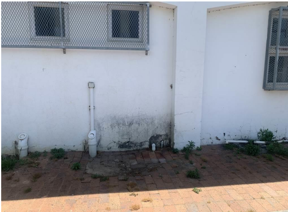
Figure 3: Some of the cracks that must be repaired at the external walls
