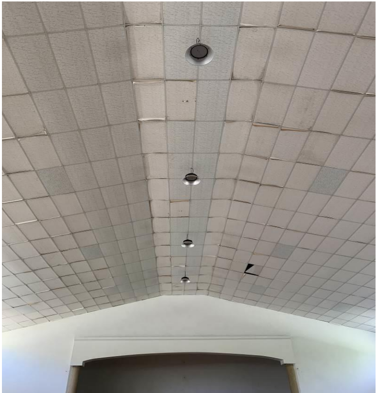
Figure 8: Ceilings in the hall area must be replaced
