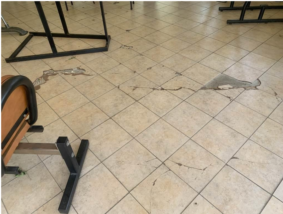
Figure 6: Floor tiles in the gym area must be removed and replaced with new tiles
