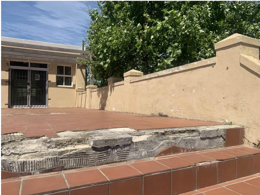
Figure 5: Tiles on the steps must be removed and replaced, walls must be cleaned and painted
