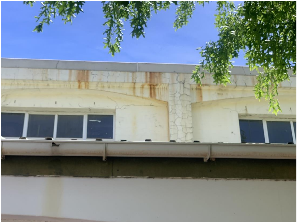
Figure 4: Crack repairs and painting that must be done
