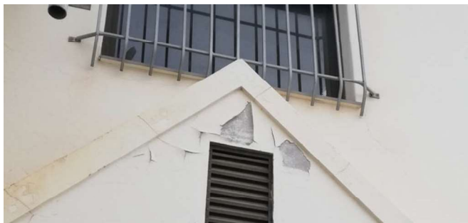
Figure 6: Paint peeling and crazing
