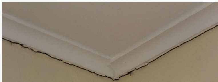
Figure 39: Delamination of ceiling cornice
