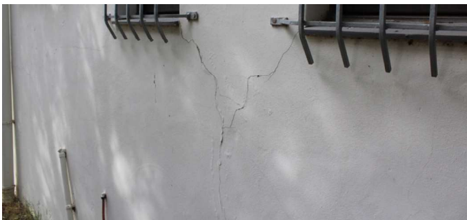
Figure 24: Crack on the wall at window opening (W10 & W11)
