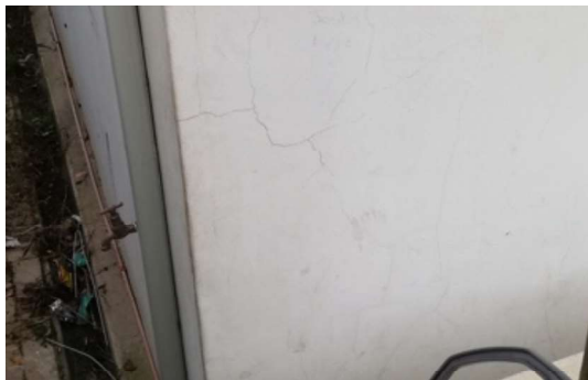
Figure 15: Cracking on wall plaster
