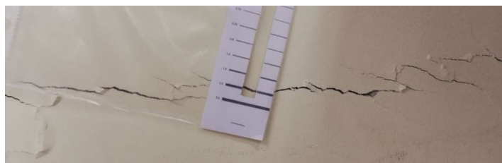
Figure 33: Close up on crack above
