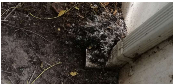
Figure 19: Blocked rainwater downpipe outlet
