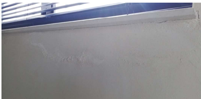
Figure 48: Damp on the wall
