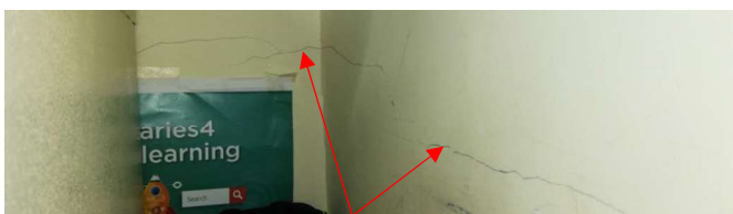
Figure 26: Interior cracks across window 08 & 09
