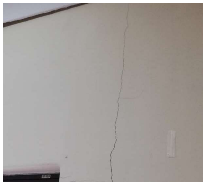
Figure 36: Vertical wall crack at entrance
