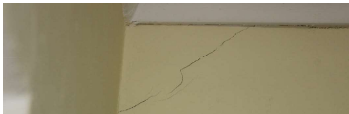
Figure 40: Wall diagonal crack below the 1st-floor slab
