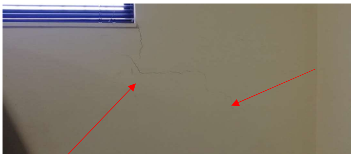
Figure 37: Crack window corner (W04)
