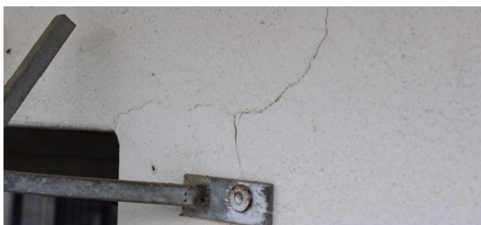
Figure 8: Diagonal crack at re-entrant corner
