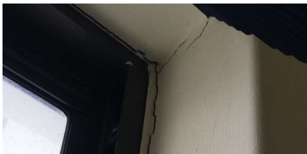
Figure 49: Cracking and separation at the door frame
