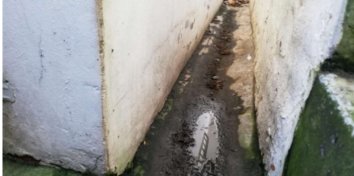
Figure 10: Ponding in the channel and horizontal crack the n wall
