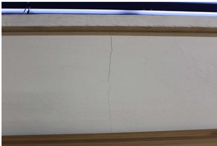
Figure 30: Vertical crack mid-span of wall opening
