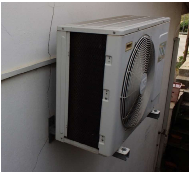
Figure 14: Vertical and angle crack behind the external AC unit
