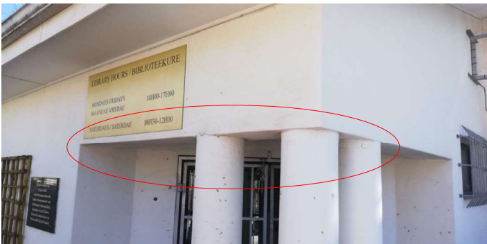
Figure 5: Cracks at the entrance
