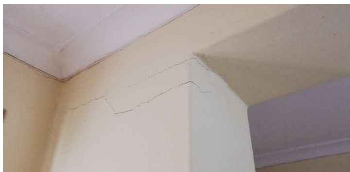
Figure 45: Horizontal crack around the brick nib
