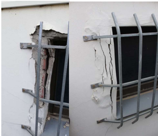
Figure 18: Cracks and plaster delamination on window reveal and jamb
