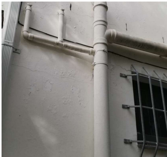
Figure 28: Horizontal cracking and paint peeling
