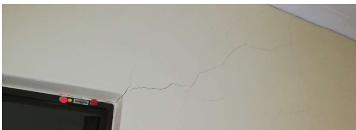
Figure 44: Diagonal crack at main council entrance
