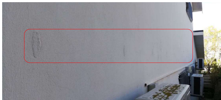
Figure 16: Crack at window corner up to the foundation
