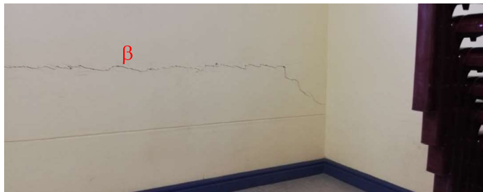
Figure 32: Crack above the structural beam
