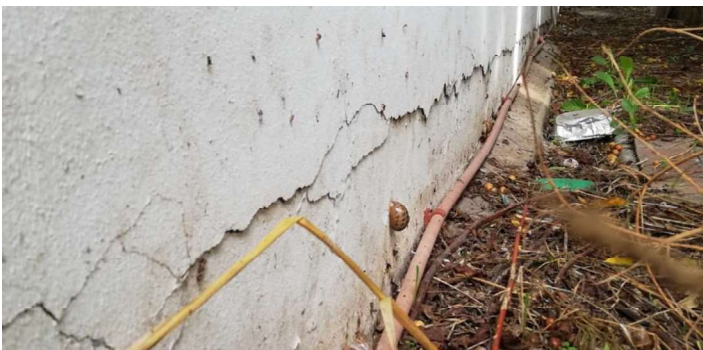
Figure 21: Horizontal crack along the entire north-west façade
