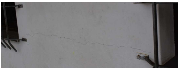
Figure 7: Horizontal crack across window openings
