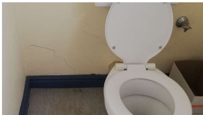
Figure 46: Crack on the gent's toilet wall
