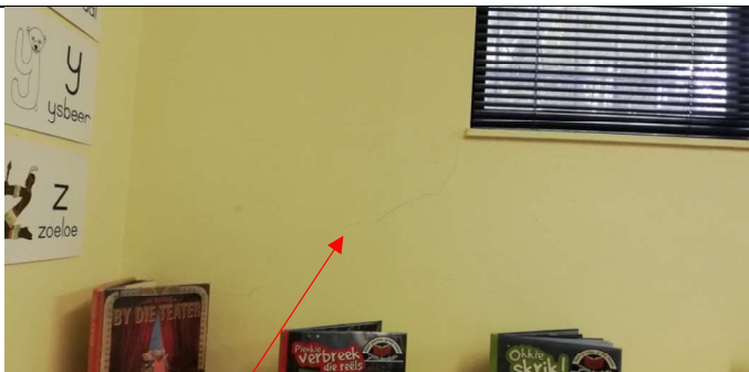
Figure 23: Diagonal crack at the window corner up to the foundation (interior)
