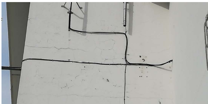
Figure 29: Cracking on the stair shaft wall
