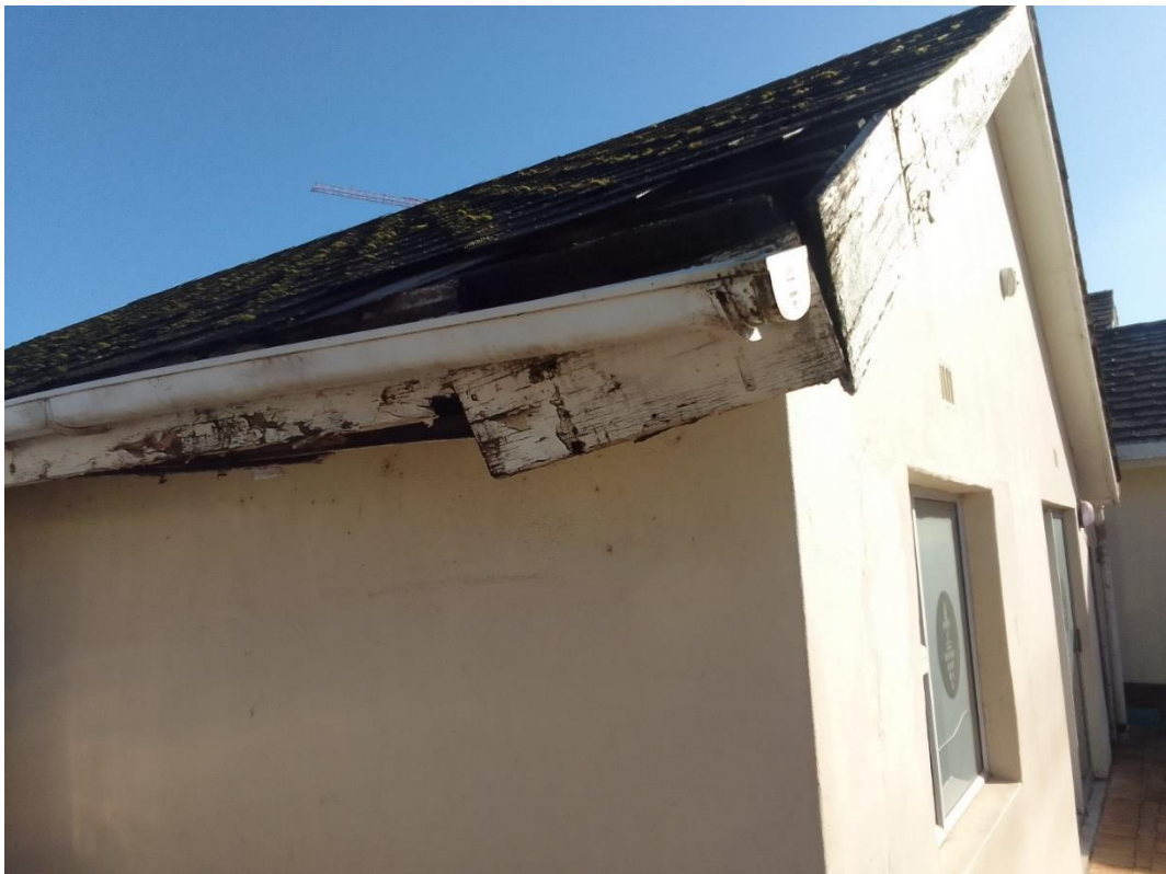
Figure 5: Photo showing condition of existing roof, gutters and downpipes.
