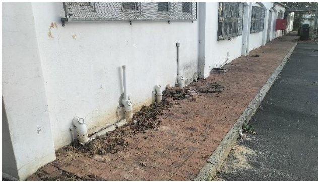
Photo 3: Paving not reinstated.
