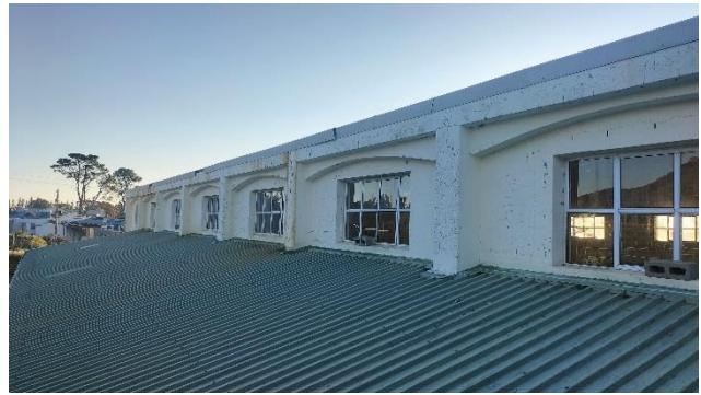
Photo 4: Signs of gutter overflowing.
