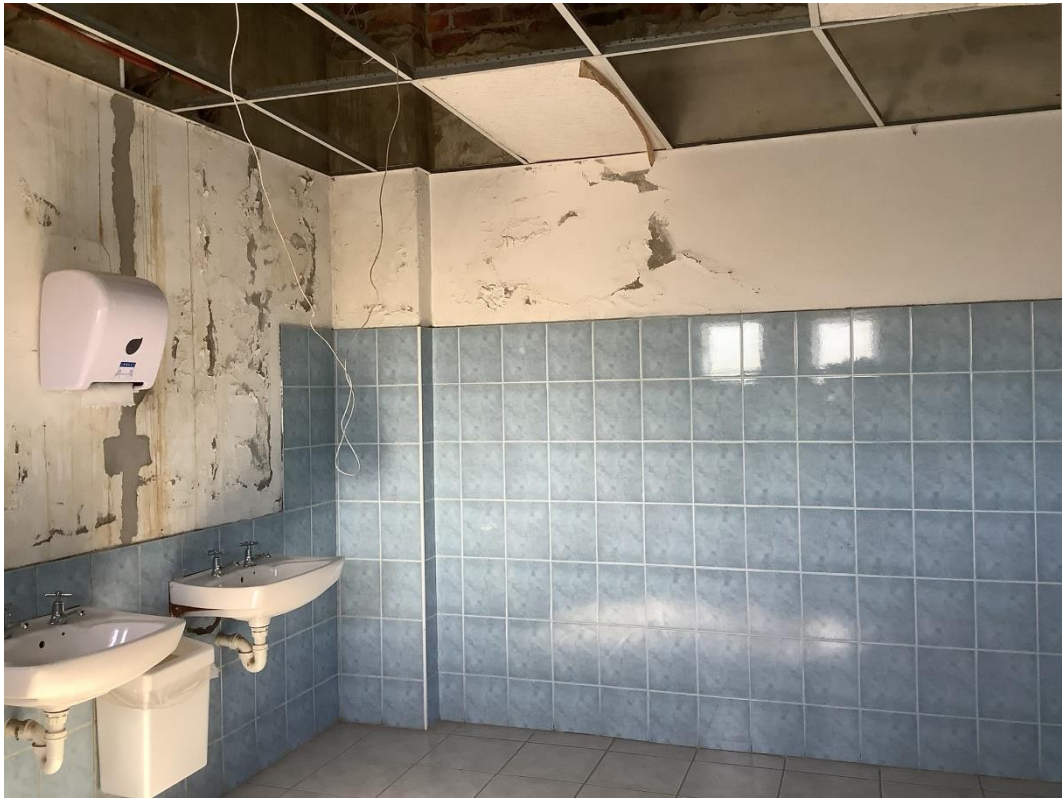
Figure 7: Photo of interior of changing room showing missing ceiling tiles and water damage to walls.
