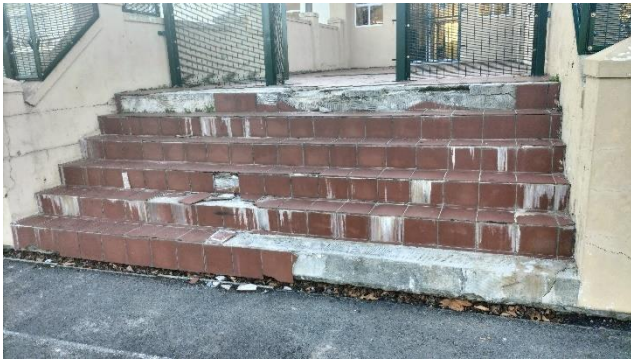
Photo 6b: Loose screed & tiles on external steps.
