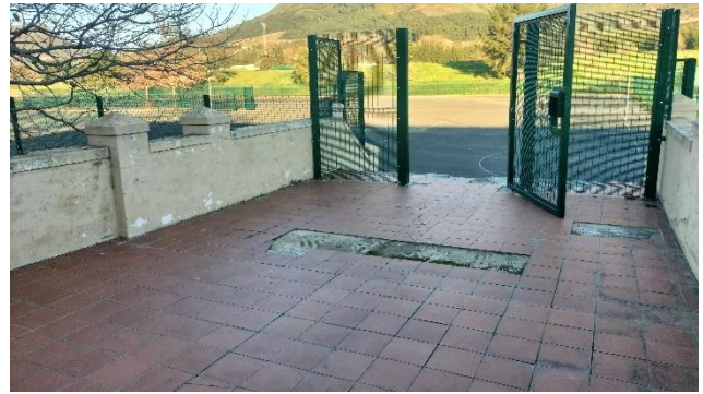
Photo 6c: Signs of ponding. Loose screed & tiles.
