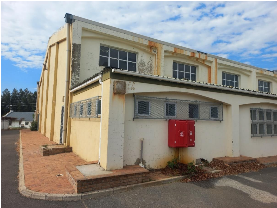
Figure 3: North-West view of building indicating water damage to façade.
