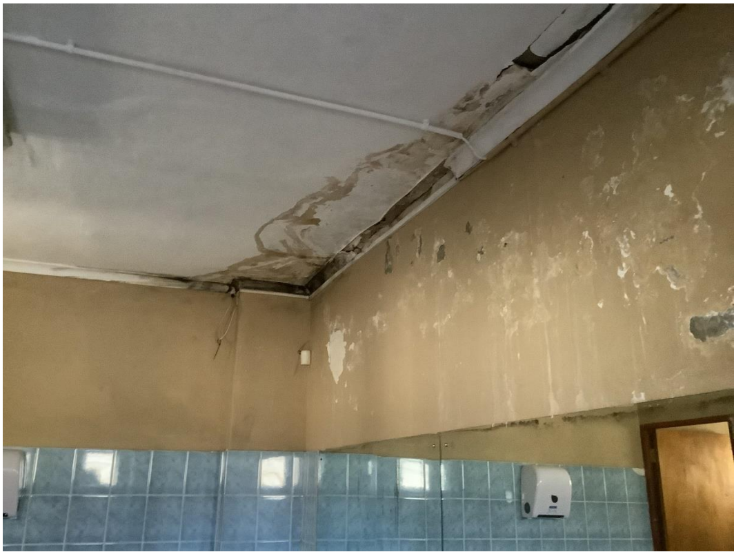
Figure 6: Photo of interior of changing room showing water damage to plasterboard ceilings and walls.
