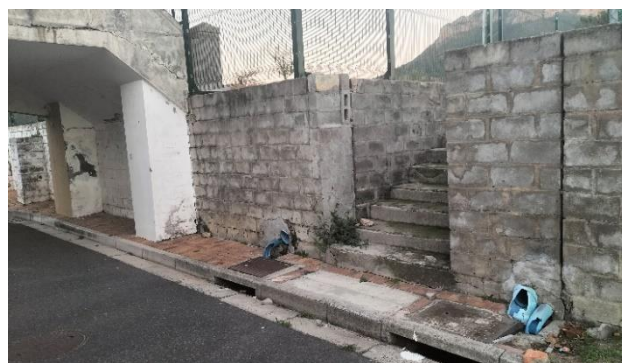
Photo 2: Damaged storm water pipes.
