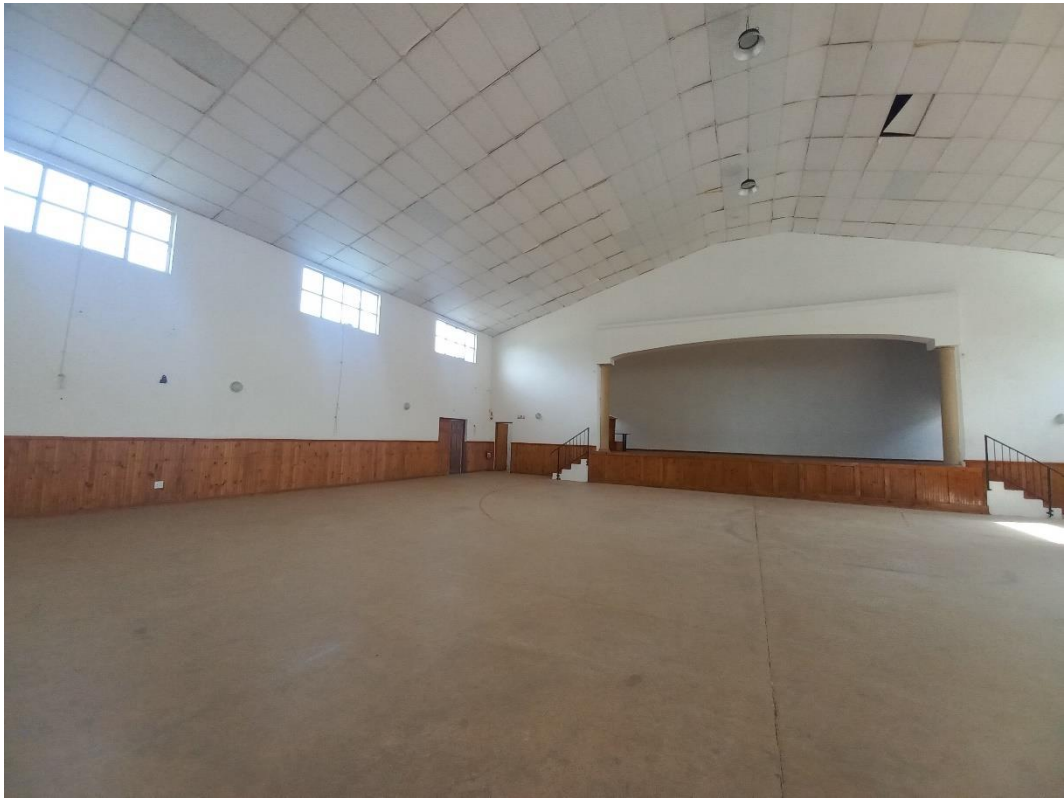
Figure 5: Photo of interior of hall showing degraded ceilings.
