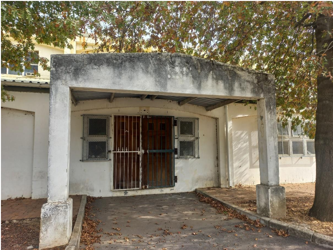
Figure 4: Photo indicating condition of external walls and plaster.
