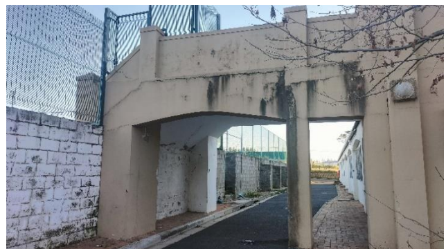
Photo 6a: External crack on face of wall.
