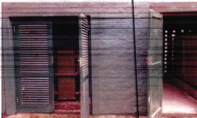
Brick built substation, no OHSA warning notices and labels, no identification of substation
