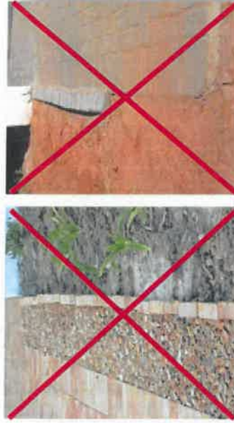
Figures 52 & 53: Incomplete and unevenly laid edging
