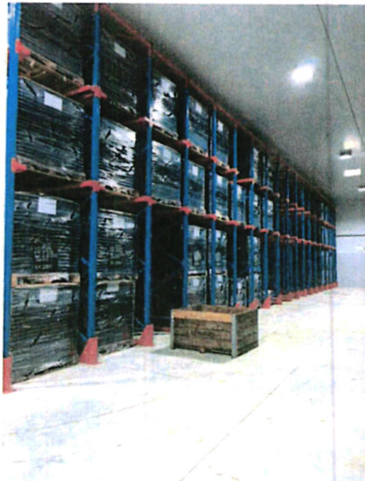
Drive in racks to be sprinkler protected.
