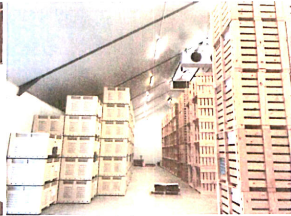
Typical block stack storage arrangement
