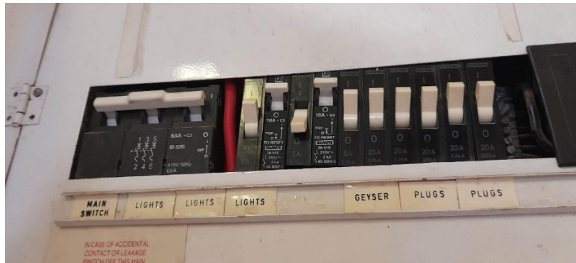
Figure 1: Main DB First row circuit breakers
