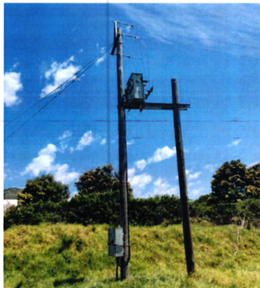
Figure 3: Existing Pump Station Transformer
