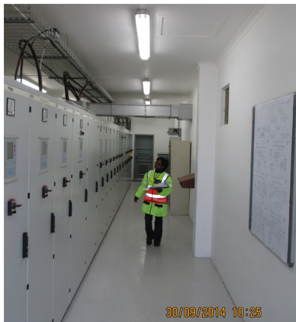
Figure 4-1 : Newly Upgraded Suidwal Substation
