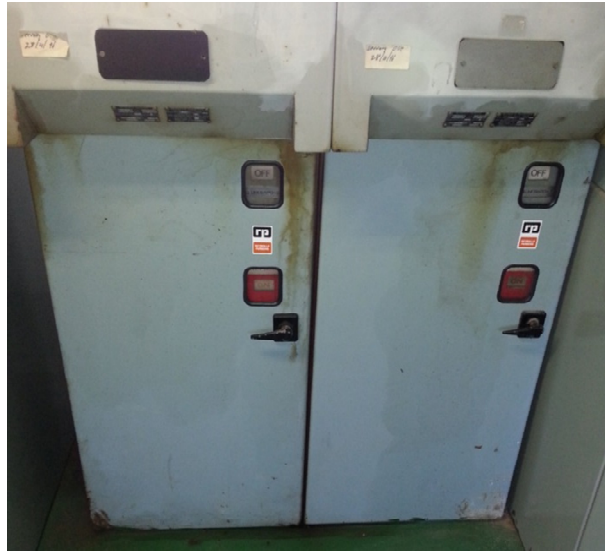
Figure 4-2 : Oil-filled Switchgear at Paradyskloof Substation
