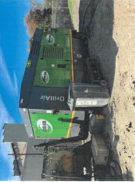
PHOTO 19: Franki-pile spill kit
