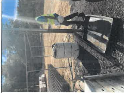
PHOTO 5: Tap and bin at site camp
