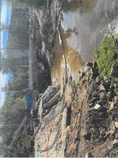
PHOTO 20: Works area – insufficient bank protection against fines washing into the river
