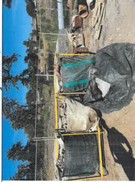
PHOTO 23: Empty cement bag waste bin storage
