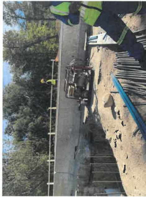
PHOTO 17: Gen set supplied with drip tray and fire extinguisher
