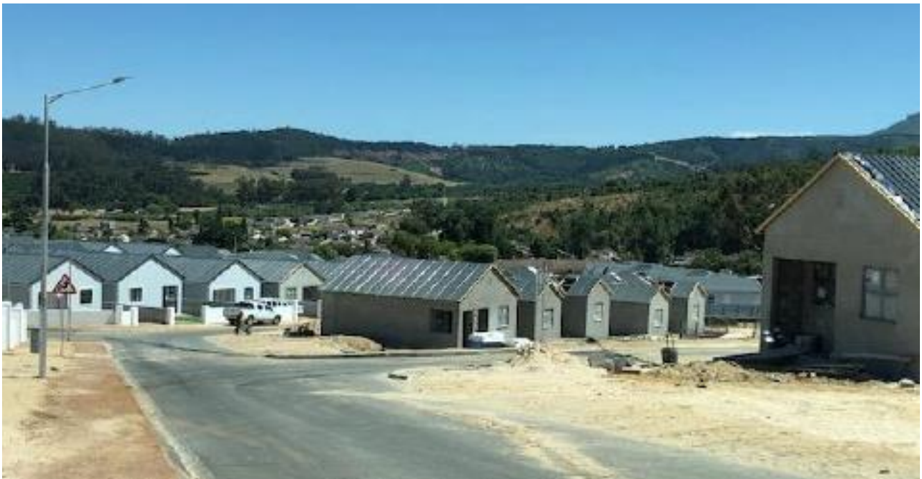
Figure 3:25: Figure 17: Work in progress on Erf 11330, Ida's Valley with the construction of GAP houses.
