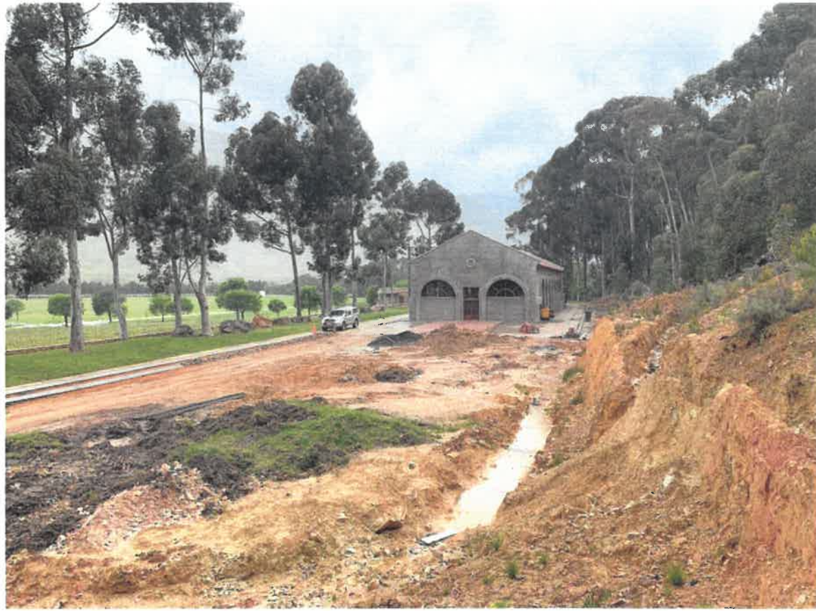
Northern aspect of the Festival Hall with the parking area under construction
