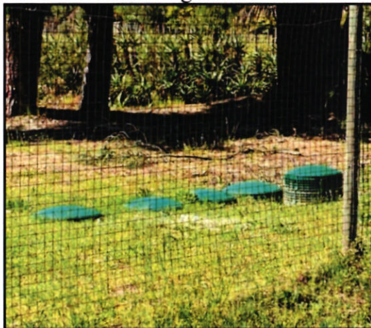
A component of the sewerage treatment system
