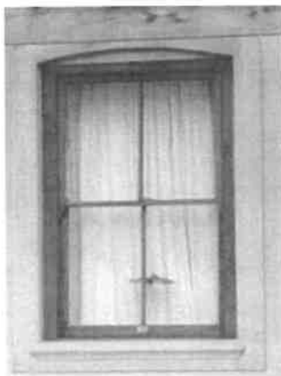
Figure 32: Plastered window sill Plaster band forming flat arch above window will be permitted
