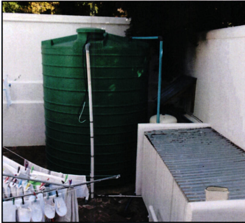
Water storage tank fed from an on-site borehole
