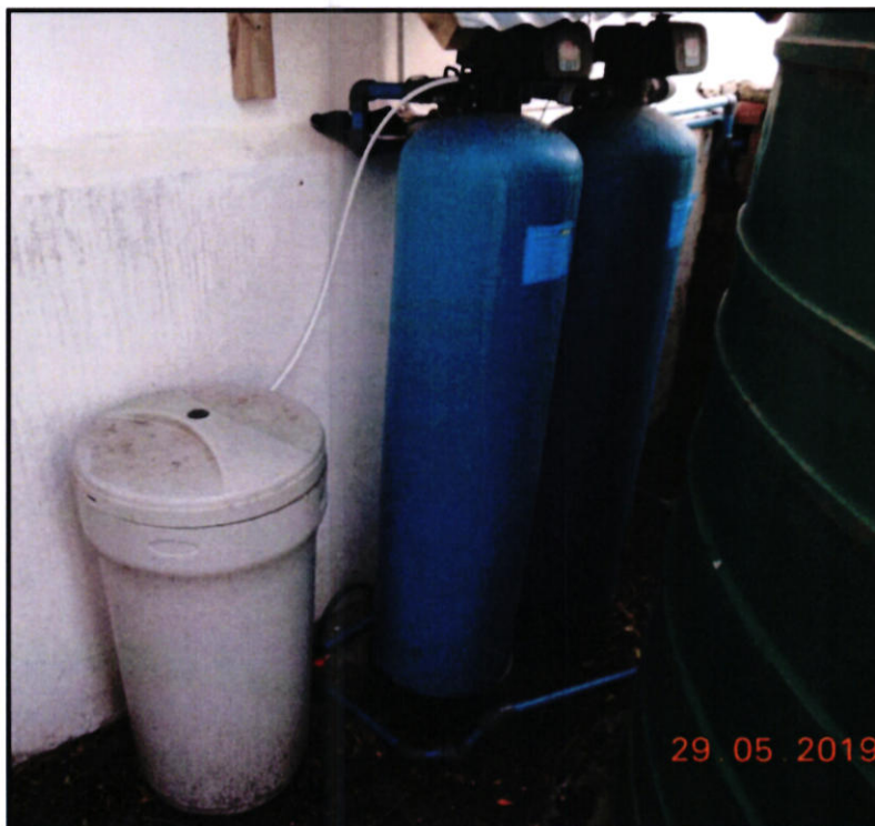
Part of the filtration/purification system
