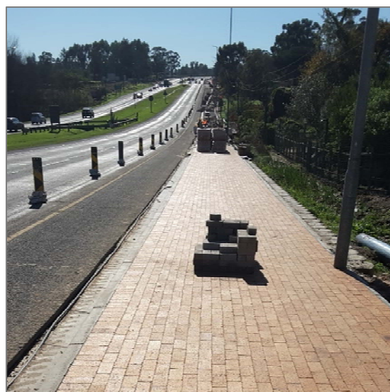
Figure 27: Jamestown: Recent upgrade of the NMT route along the R44 to the CBD
