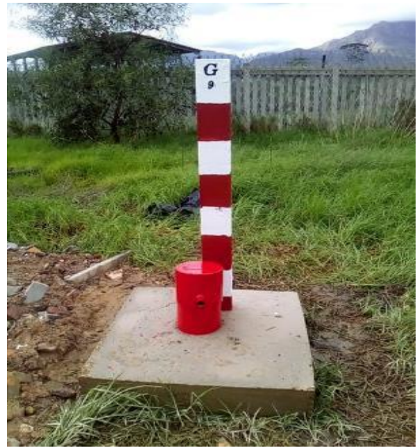
Photo: One of the installed gas monitoring wells
