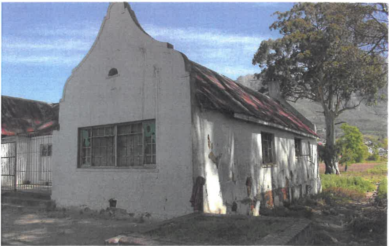
Dilapidated building on a Mixed-Use site in Lanquedoc: Erf. 32 Lanquedoc
