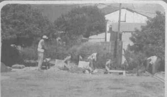
Streets were paved in Wemmershoek thus putting an end to dust clouds in summer and mud pools in winter.
