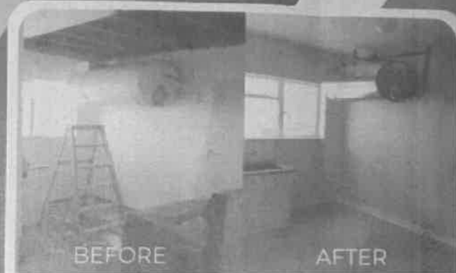
Municipal flats in Cloetesville are being upgraded into bright and airy homes.
