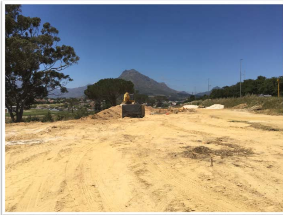
Photo 2: Erf 81/9 in an easterly direction
