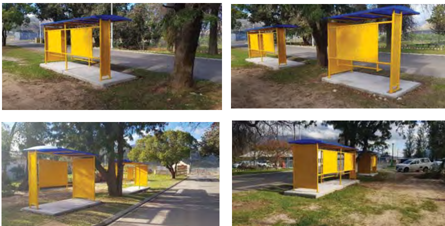
2 No. shelters installed in Wemmershoek (close to the R301 Road in Angelier Street.)
