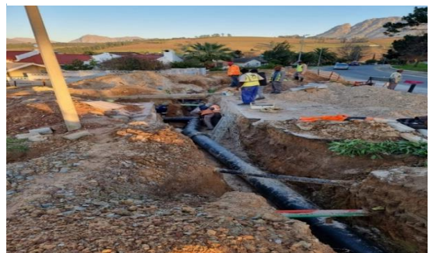
Figure 43: Vlottenburg New Outfall Sewer (Longlands)
