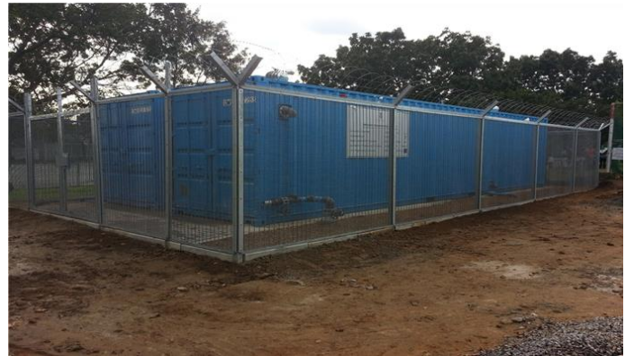
Figure 49: Stellenbosch Containerised WTW – Van der Stel
