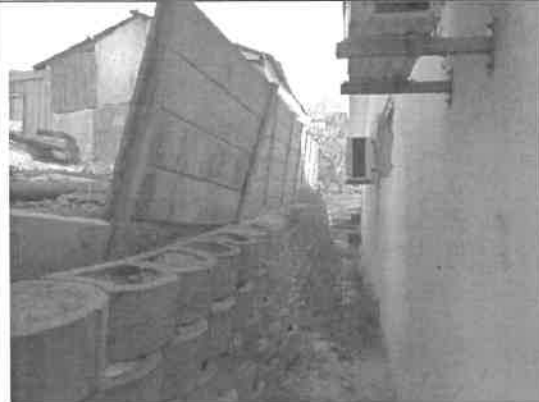
Clear view of vibracrete slabs missing and wall foundation shift. More follow up is needed.
