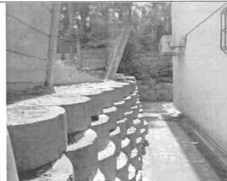
Compared with picture above its clearly visible that the Base of retaining wall has shifted dramatically in a space of a year.
