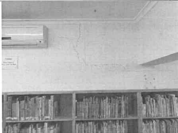
Interior of cracks emanating from cracks above from exterior. More follow up is needed.
