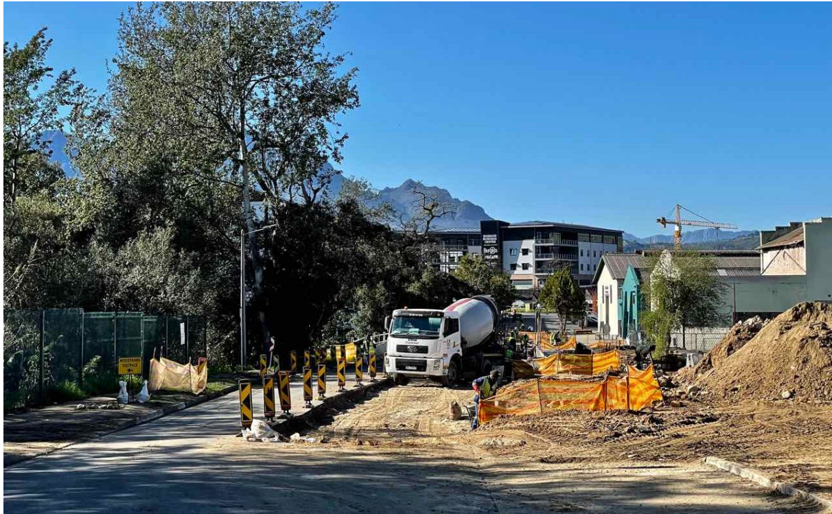
FIGURE 30: View towards the current Plankenbrug Bridge located approximately 60m north of the old bridge in Figure 29. (node 2 in Figure 01). Although some remnants of the area's rural character are still evident on the left, the precinct is steadily being transformed out of all recognition from what it once was. (Image, ARCON, 6 July 2022).
